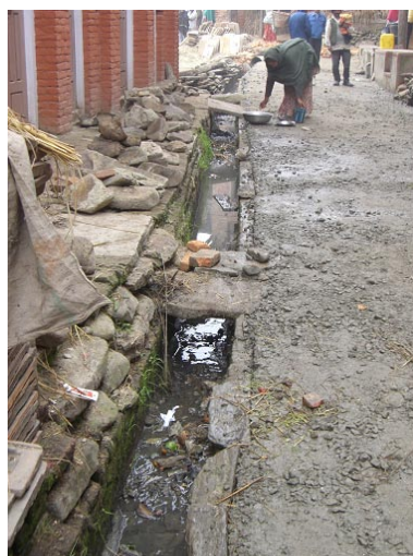
Figure 2. Drainage system in Khokana.
